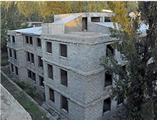
Early construction of the new Axumite Heritage Foundation Library and Cultural Center
