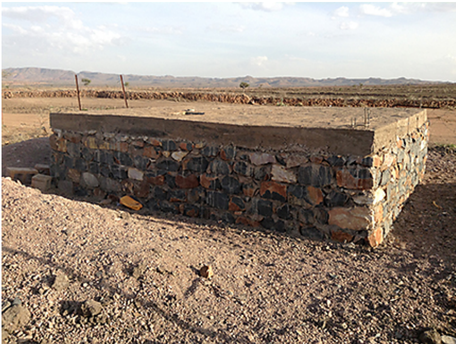
The concrete and rock structure slightly above ground is the final foundation for the Preparatory School. The School will continue
