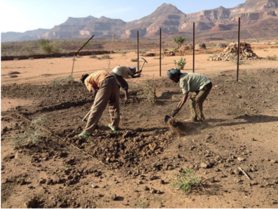
With mountains behind them, workers are digging a very shallow hole that is the beginning of the Preparatory School's latrine foundation.
