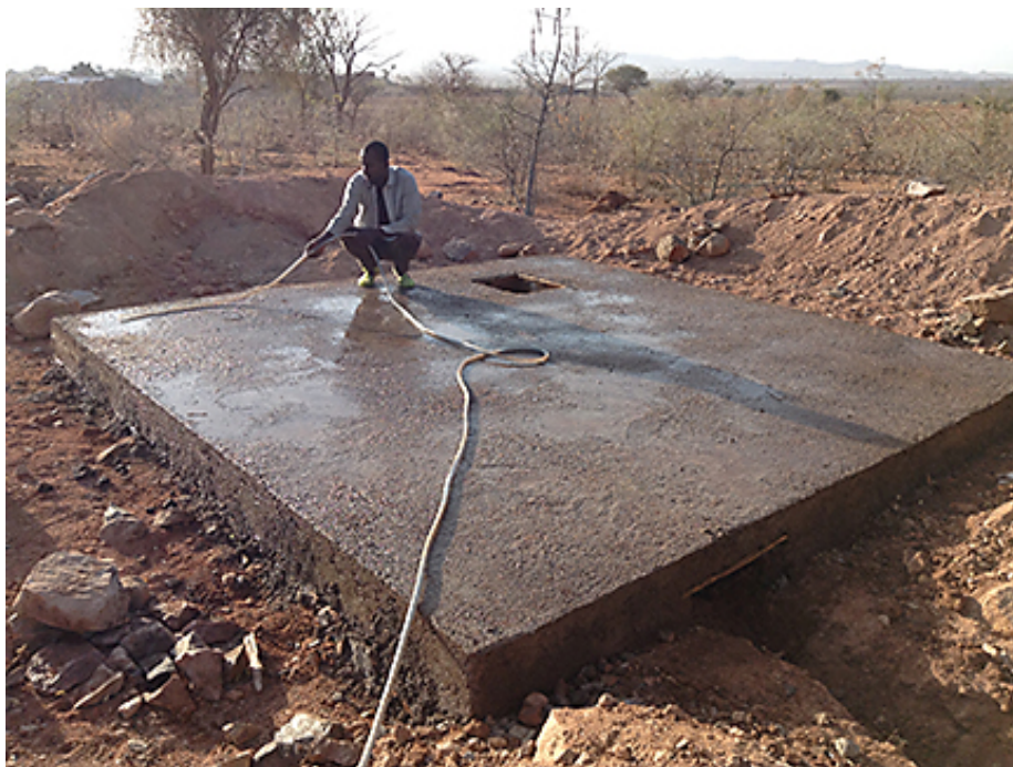
The concrete slab being watered is the final completed foundation for the Secondary School. Note in the lower right a trench leaving the hole.
