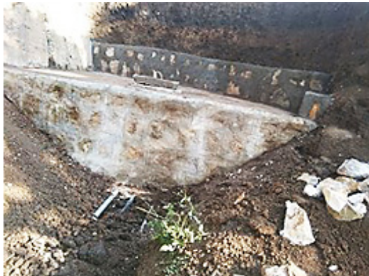
Water distribution point
